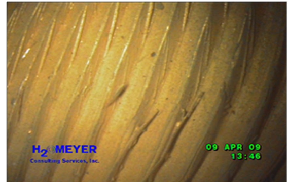
Row 15, Tube 24 – Manufacture defects of the tube enhancements
