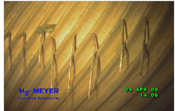
Row 30, Tube 41 – Manufacture defects of tube enhancements
