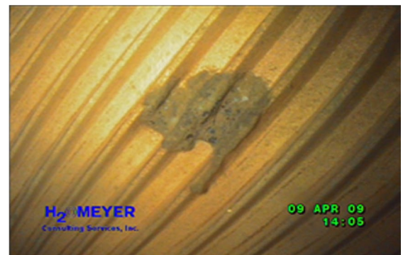
Row 30, Tube 41 – Visible corrosion
